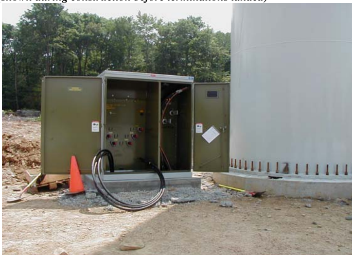
Typical Pad-Mount Transformer (shown during construction before terminations landed)
