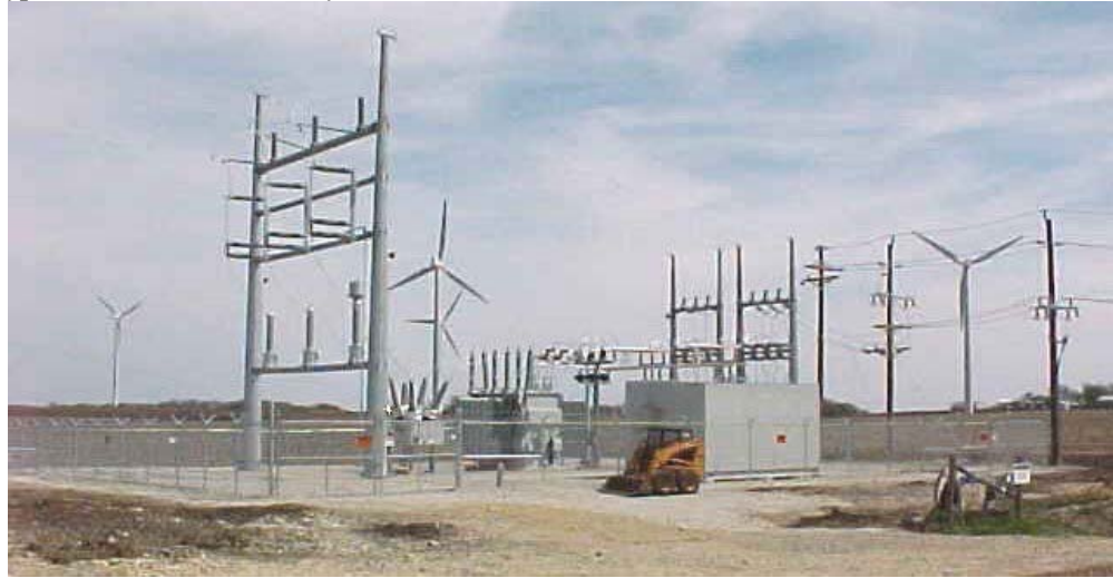
Typical Wind Power Facility Substation
